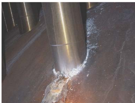
Nozzle leakage on the reactor vessel head at Oconee led to inspections at other plants.
